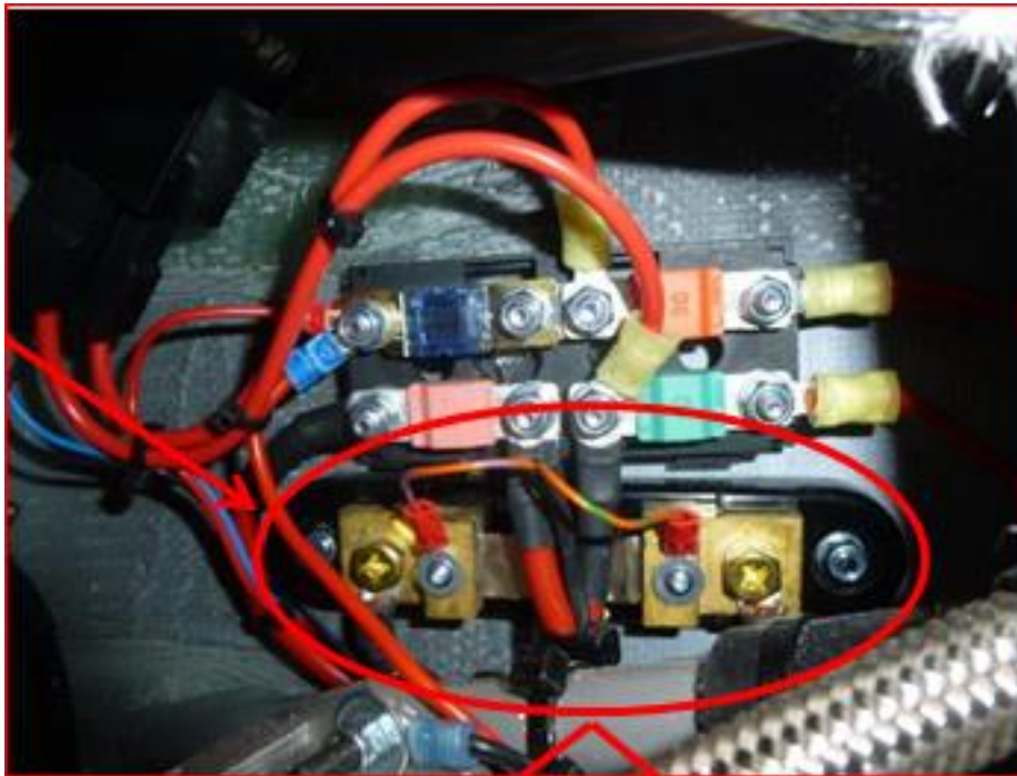
Fig 1: Shunt, old installation
